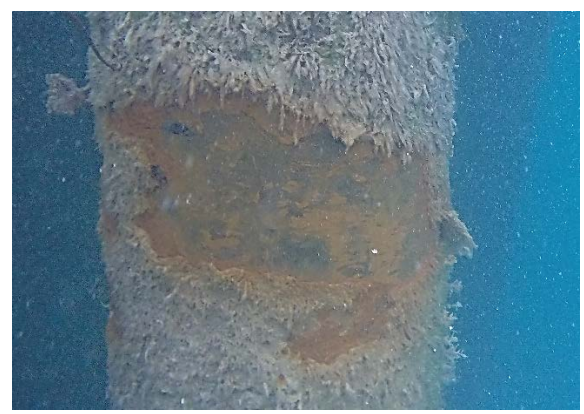
Fig. 3hh - Band of extreme corrosion, H-MD2
