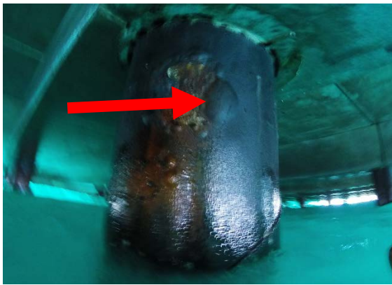
Fig. 1r – Blisters on protective coating in splash zone
