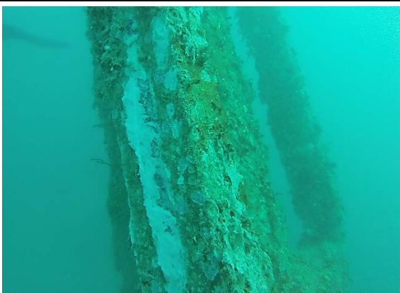
Fig. 3i - Anode of walkway dolphin, more corroded than others
