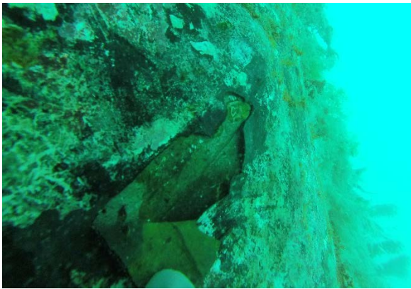
Fig. 2a Protective layer peeled away to show steel underneath, Pile 158
