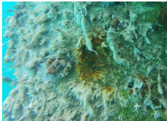
Fig. 1i - Typical example of ALWC on pile surface
