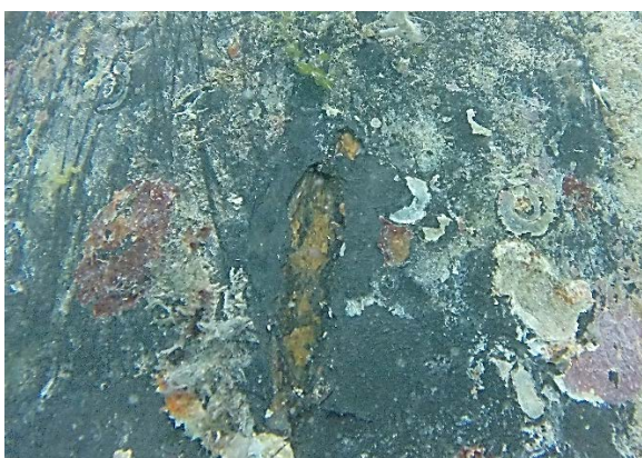
Fig. 3k - Steel exposed under protective layer, H-MD4
