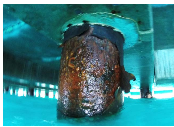
Fig. 1u Compromised protective coating and corrosion
