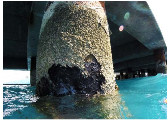
Fig. 2f – Extreme example of corrosion in splash zone
