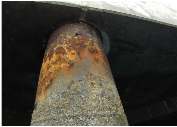
Fig. 1j – Compromised protective coating and corrosion in splash zone
