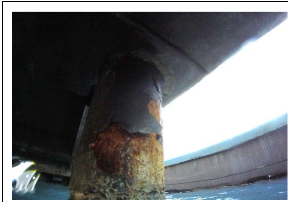
Fig. 1v – Coating peeling away
