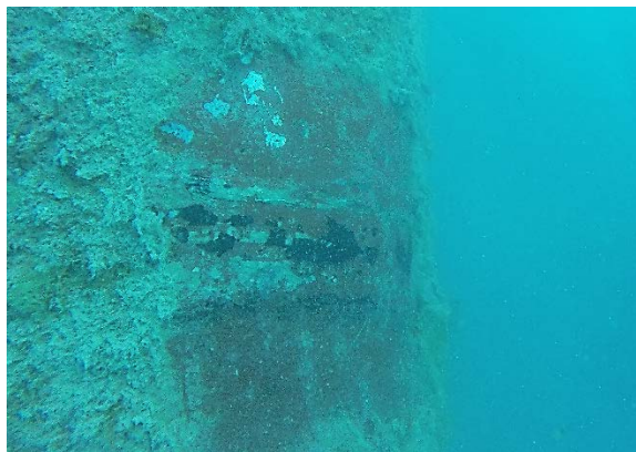
Fig. 3e - 1 st Level 2 inspection, HMD6, very minor surface corrosion
