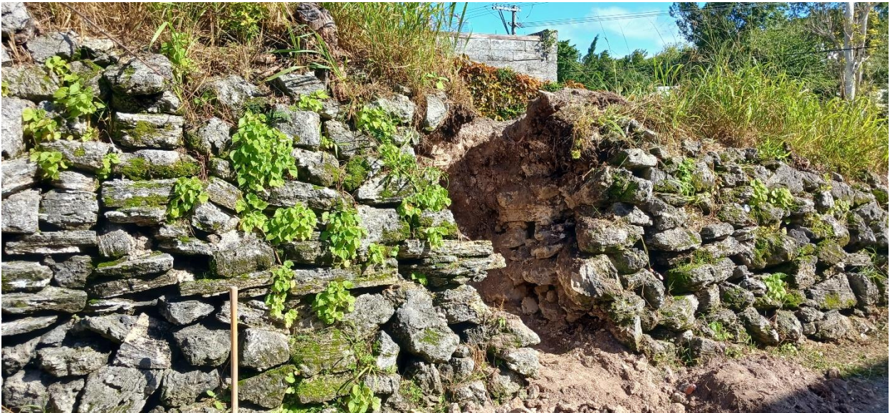
Figure 2 - Further view of investigation. No sound rock was found, only fill material and dry stack.
