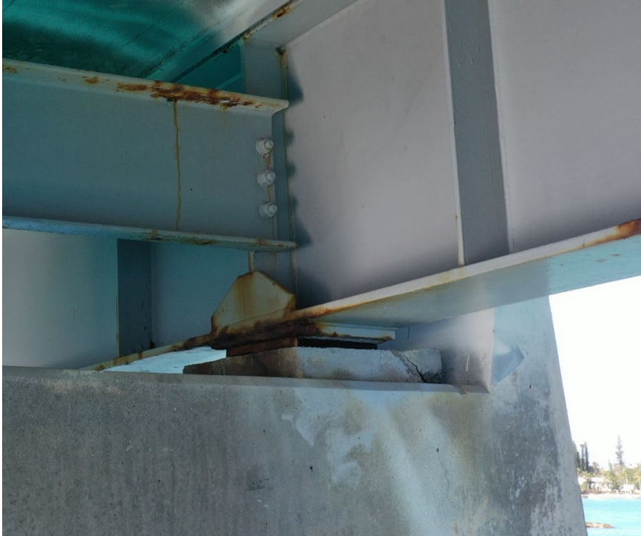
Photograph 9 – Bearing B12 showing local cracking on the edge of concrete plinth.
