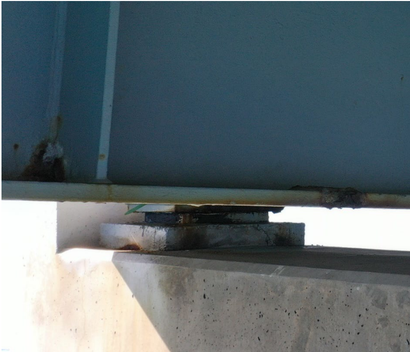
Photograph 7 – Bearing B9 showing vertical and diagonal cracking.
