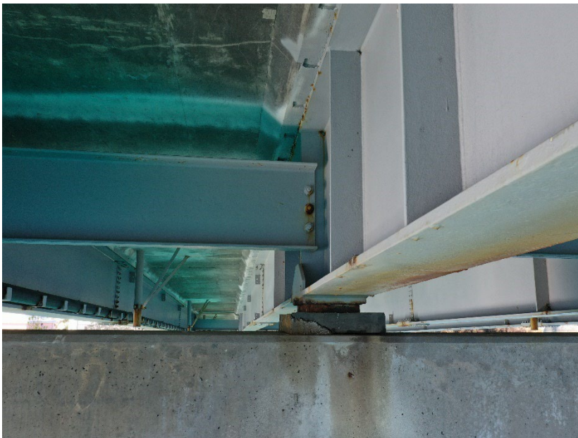
Photograph 8 – Bearing B10 showing a diagonal crack.
