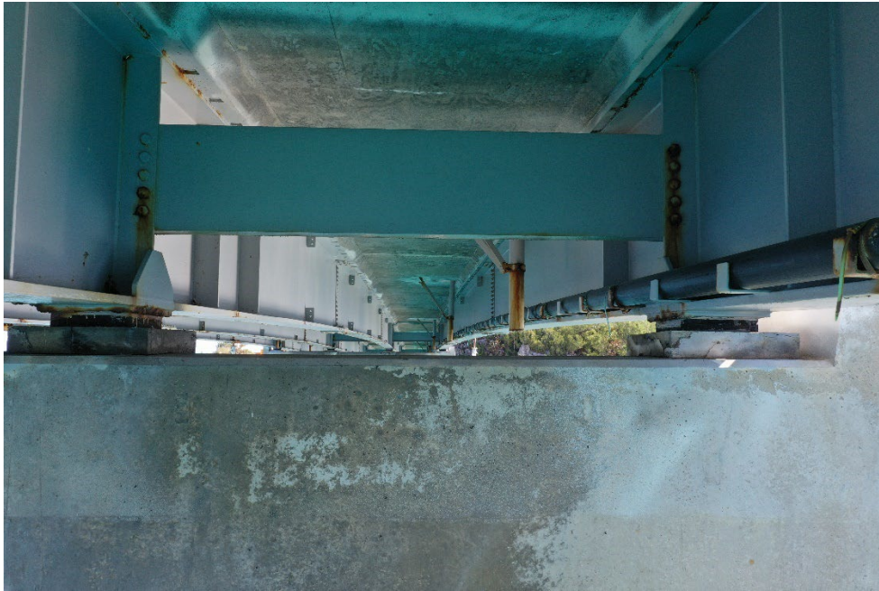
Photograph 11 – Bearings 13 and 14 showing cracking of the concrete plinths.
