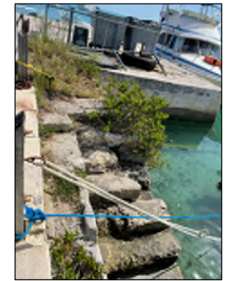
6 VEGETATION AND DAMAGED STAIRS
