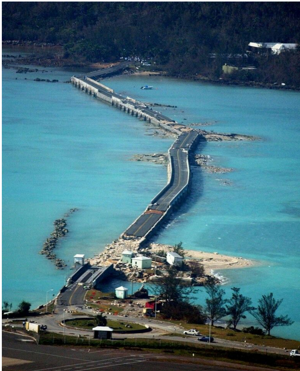
Figure 9.10 Damage sustained to the Causeway during Hurricane Fabian in 2003
