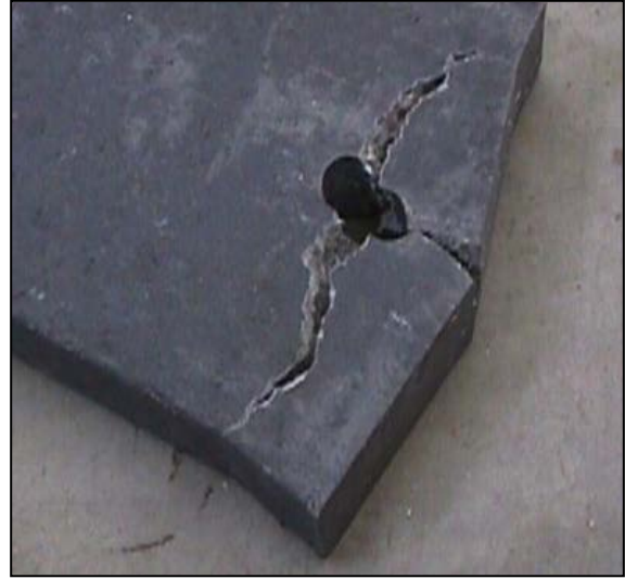
Figure 3-39 Failure of Composite Member
