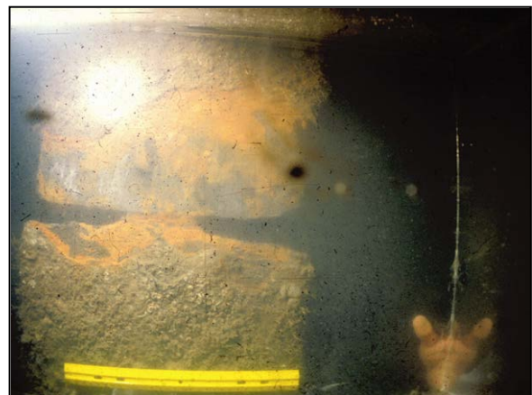
Figure 3-27 H-pile Corrosion Below Concrete Encasement
