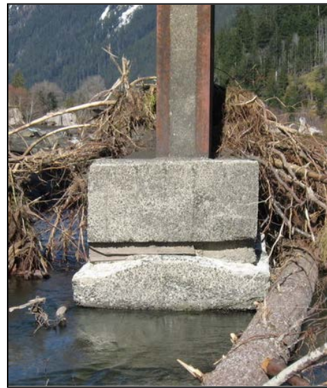
Figure 3-14 Foundation Seal Under Pier Exposed by Scour
