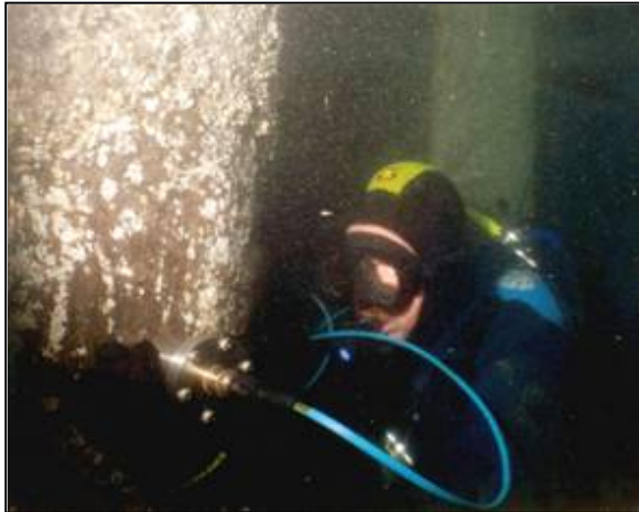
Figure 5-9 Diver Applying the Transducers to a Pile for the Direct Transmission Method
