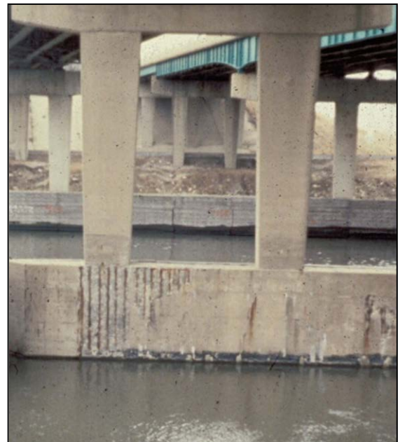
Figure 3-23 Spalling of Concrete at Waterline
