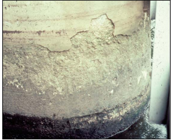
Figure 3-22 Scaling of Pier at Waterline
