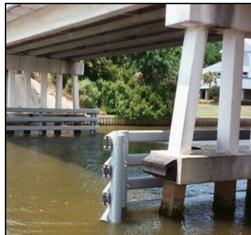
Figure 3-8 Composite Pile and Wale Fender System
