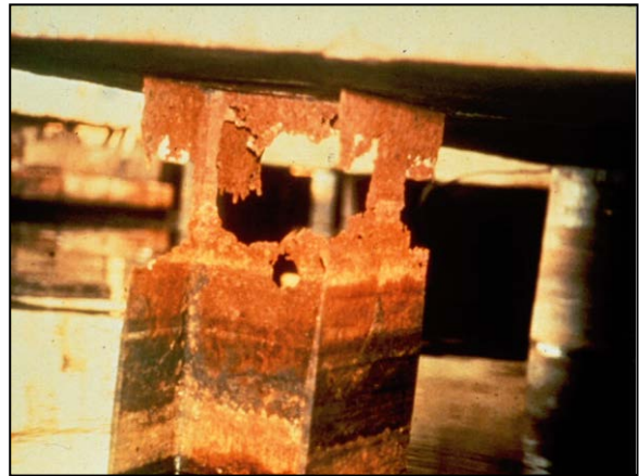
Figure 3-26 Severely Corroded H-Pile
