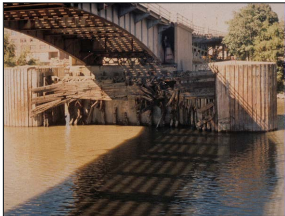
Figure 3-17 Timber Fender System Attached to Pier with Steel Sheet Pile Cell Dolphins
