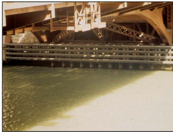
Figure 3-18 Pile Supported Fender System
