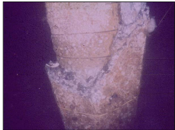
Figure 3-25 Pile Damaged by Delayed Ettringite Formation
