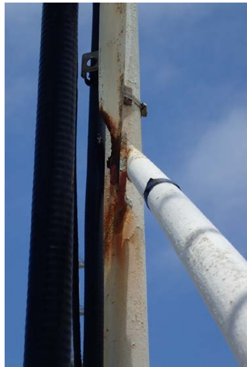
Tower surface condition File 124
