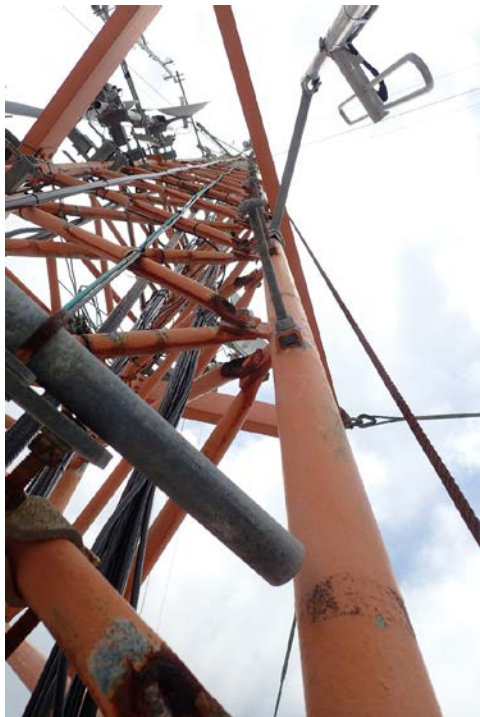
Tower surface condition File 079
