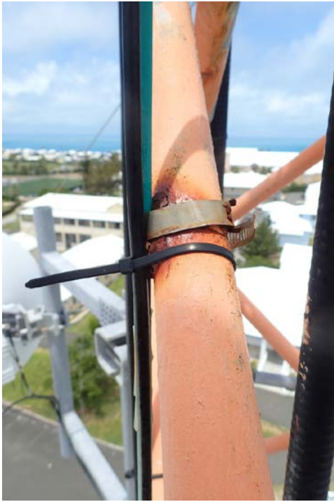
Tower surface condition File 129
