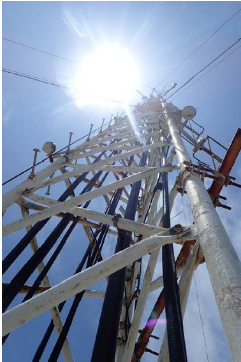
Tower surface condition File 113
