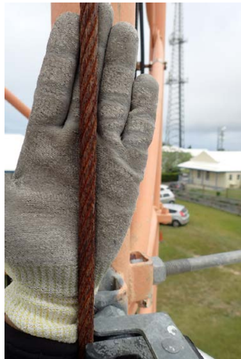
Safety cable condition File 048
