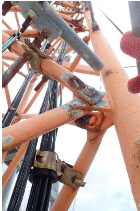
Antenna #10 stiff arm connection to damaged diagonal File 078
