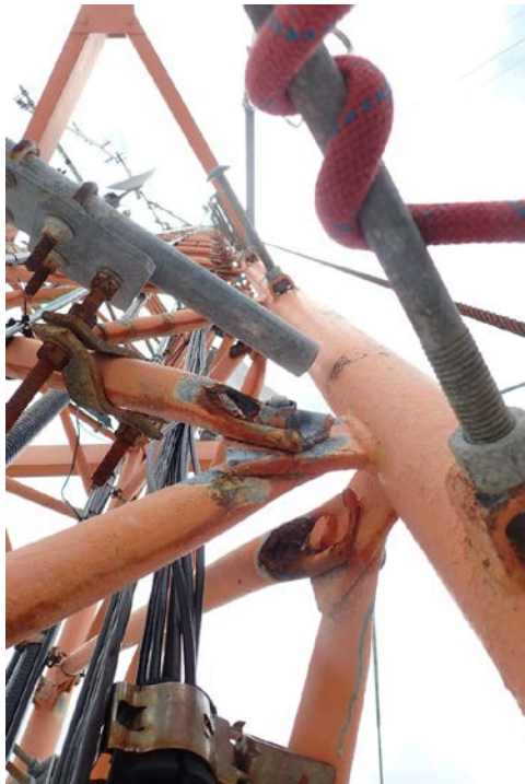
Antenna #10 stiff arm connection to damaged diagonal File 077
