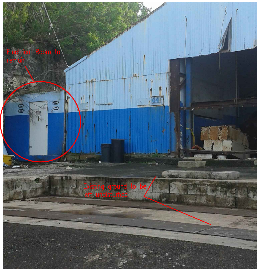
FRONT VIEW ELECTRICAL ROOM
